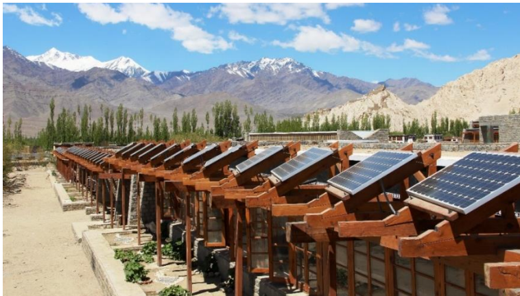
Figure 26 Photo voltaic panel installation where the panels also provide shading to glazing
